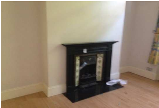
Photo 21 First floor - Rear (F 01) Fireplace number: FF01 Comments: Inappropriate fireplace
