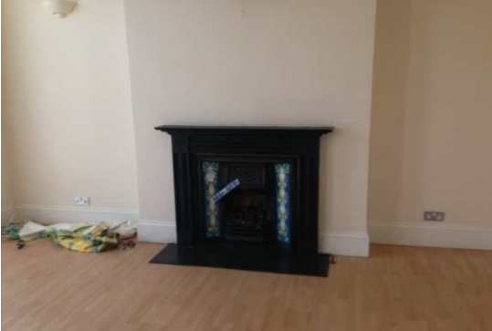
Photo 19 First floor - Front (F 02) Fireplace number: FF02 Comments: Inappropriate fireplace
