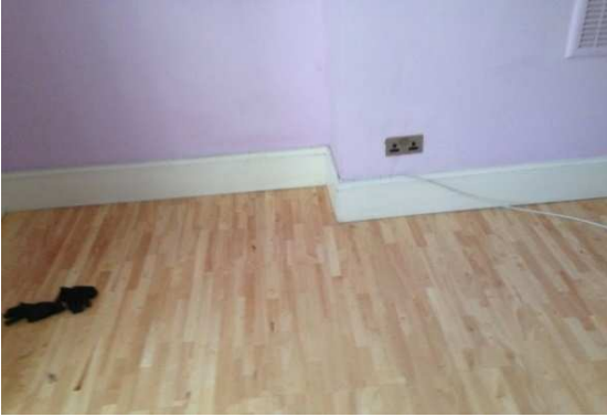
Photo 15 Ground floor - Front (G 02) Fireplace number: GF 02 Comments: Non existent Blocked in
