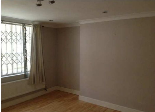
Photo 13 Lower Ground Floor - Front (LG 04) Fireplace number : LGF 01 Comments: Non existent, Blocked in
