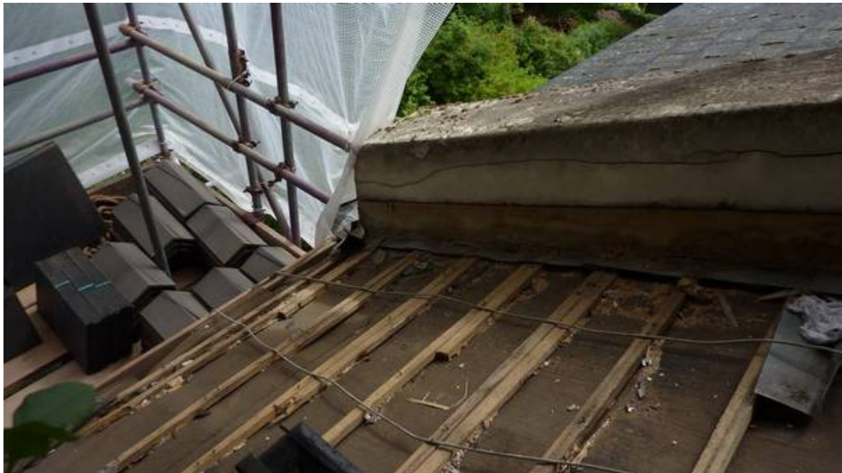
(1) Existing parapet wall to the rear of the property looking towards the eaves
