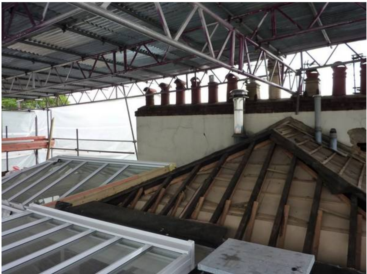
(5) Severely cracked render to the chimney stack on to the rear of the property
