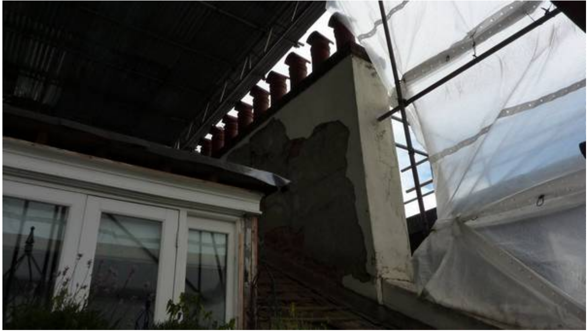
(4) Damaged render and exposed brickwork to the chimney stack on the street side of the property
