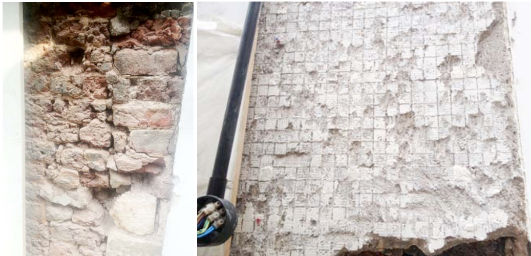
Infill brickwork and lost facings
