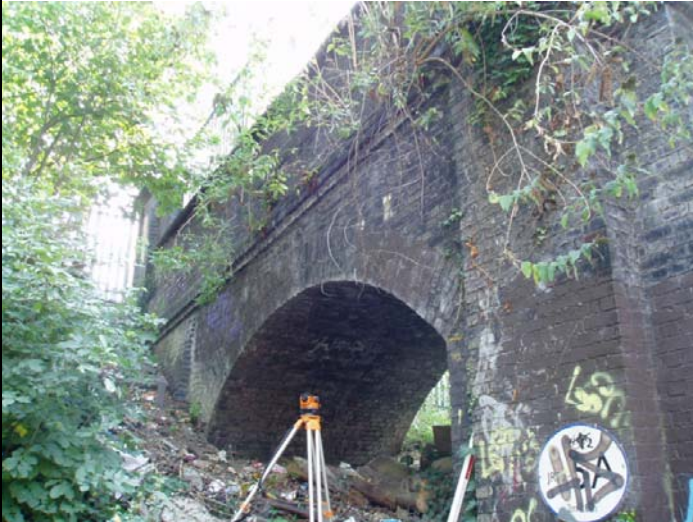
Defective Brickwork, South East Arch Elevation
