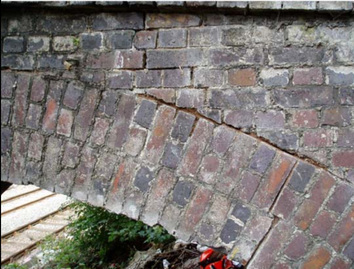
Defective Arch Brickwork Profile.
