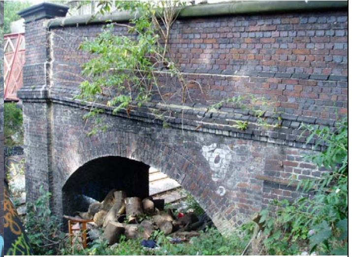
Defective Brickwork, South West Arch Elevation
