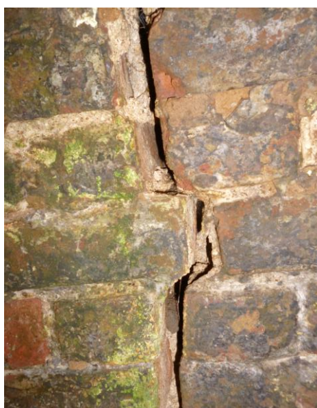
Plate 3.6: Example of cracks in the brickwork
