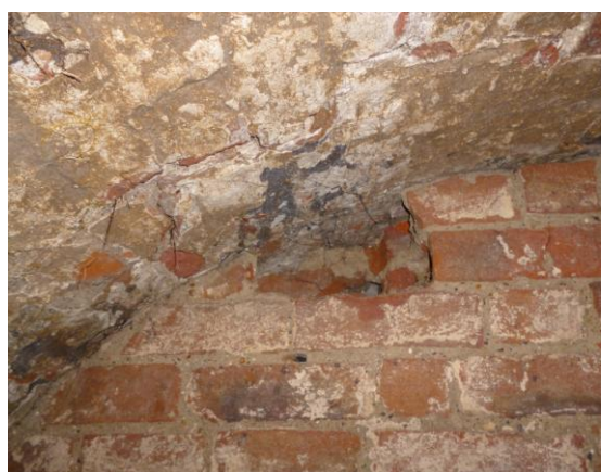
Plate 3.7: Example of cavity within brickwork of the tunnel
