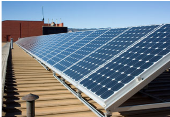
Figure 4 – Example roof mounted monocrystalline array
