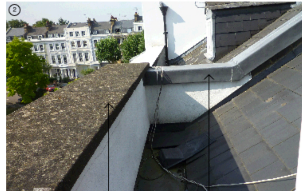
damaged cornice to be repaired
