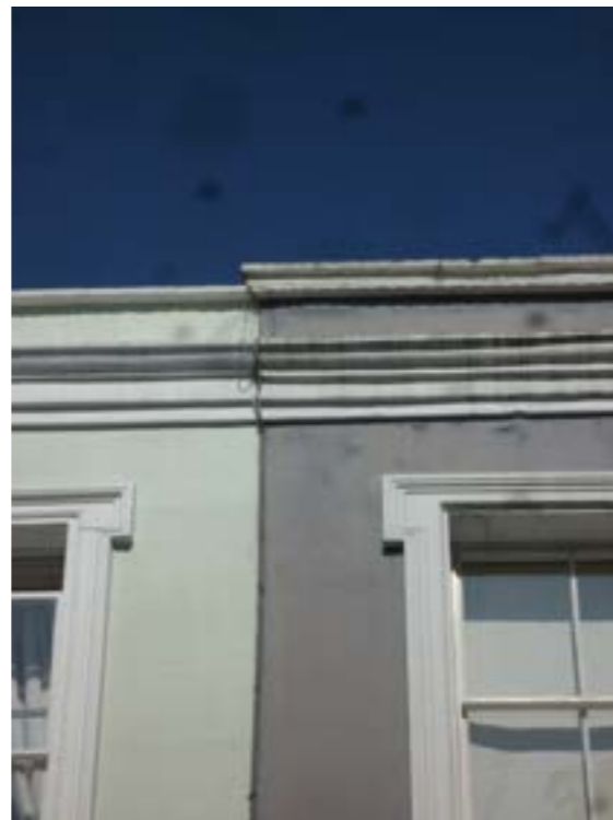
Existing mis-alignment of the parapets to 32 Chalcot Square (left) and 31 Chalcot Square (right)
