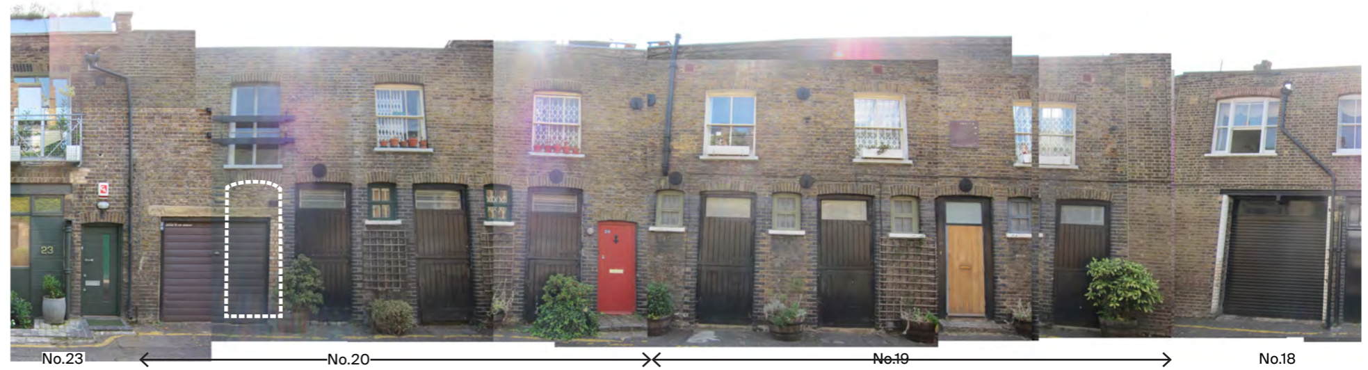
Photograph of existing elevation. Dotted line indicates location of proposed reinstated opening.
