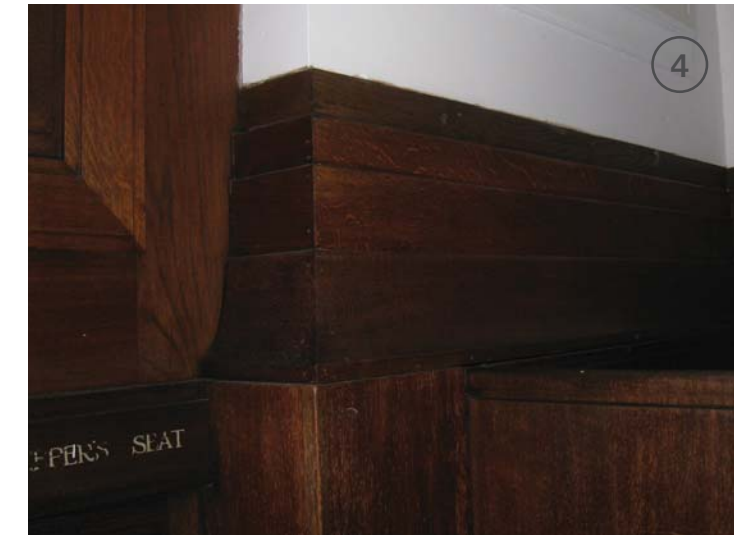
Existing timber panelling to be retained. Timber nosing to steps to match existing panelling to provide contrast with treads and risers.
