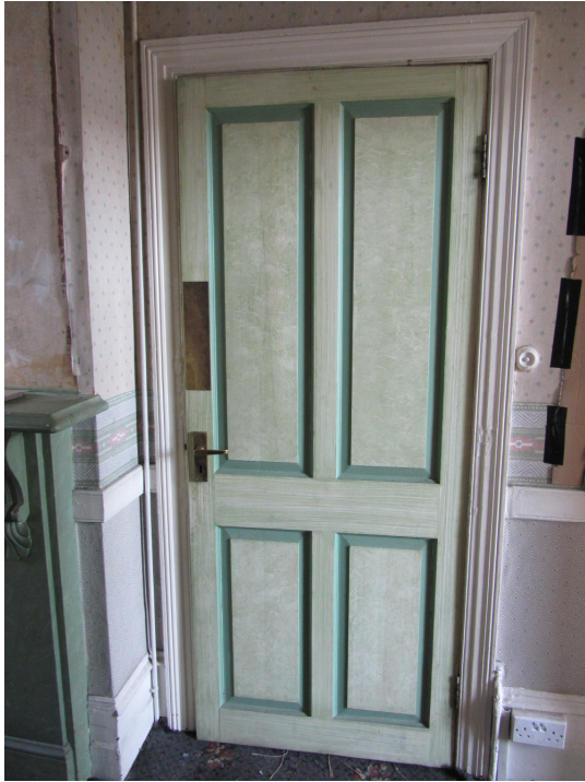
Door Type 'X' modern poor quality 4 panel door
