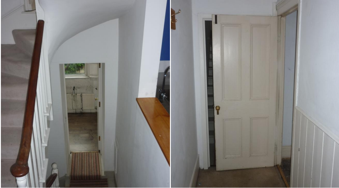
Above left: first half landing: ply faced and modern door to room off landing Above right: ground floor, front room. Original looking but in fact softwood sections and mouldings applied to a ply back. Likely original style of door and used as basis for proposals.
