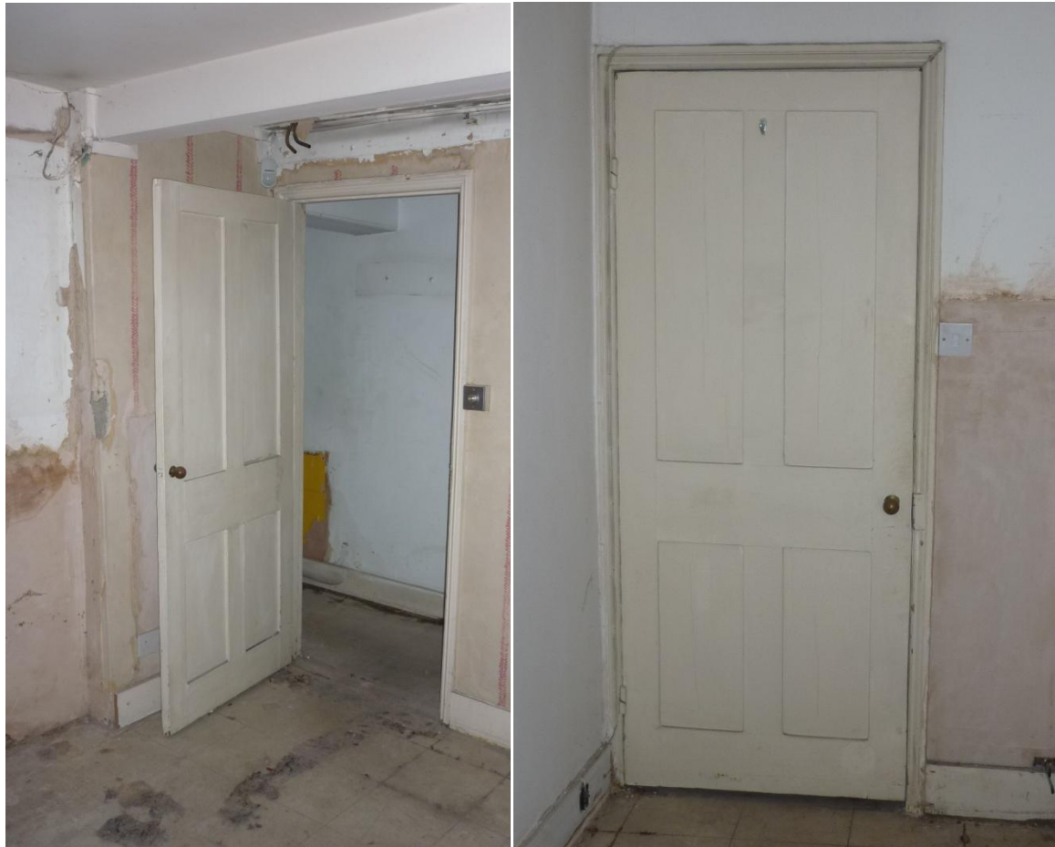
Above left and right: the two basement bedroom doors, both of which are original, and will be retained.
