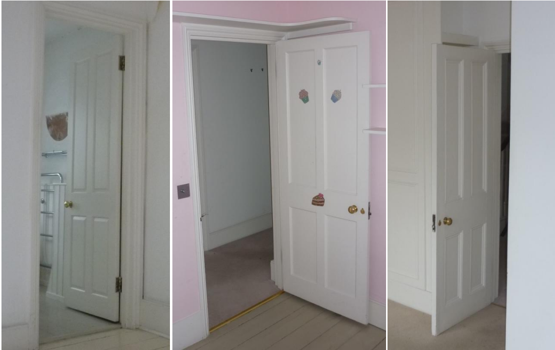
Top left: third floor bathroom: hollow core 4 panel wood effect door (same as door to top stairs on third floor)
