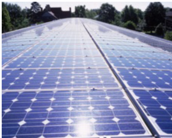
HORIZONTAL SOLAR PANELS
