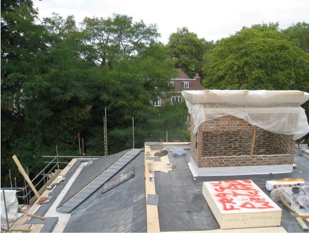
PH05 Brown roof to North of Proposed Terrace to become Green roof.
