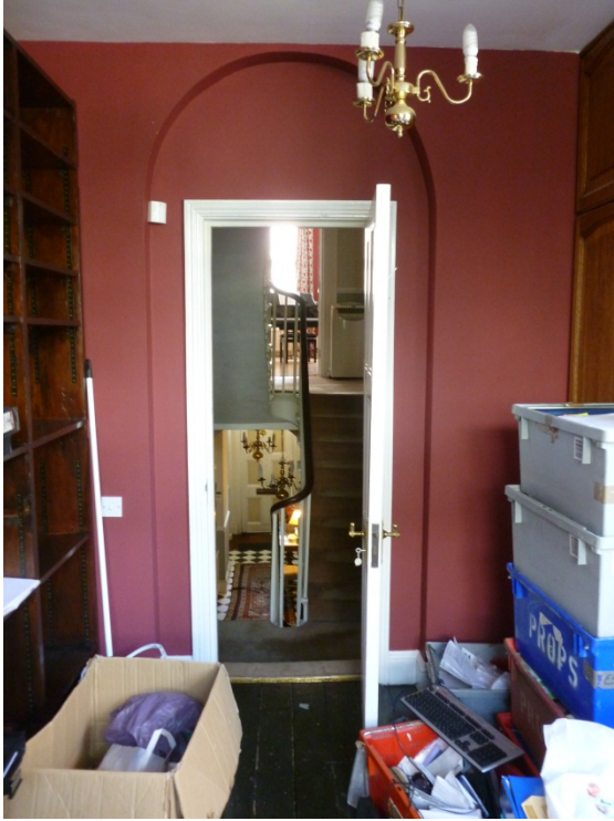
Existing first floor door and surround to be removed to reveal original opening.
