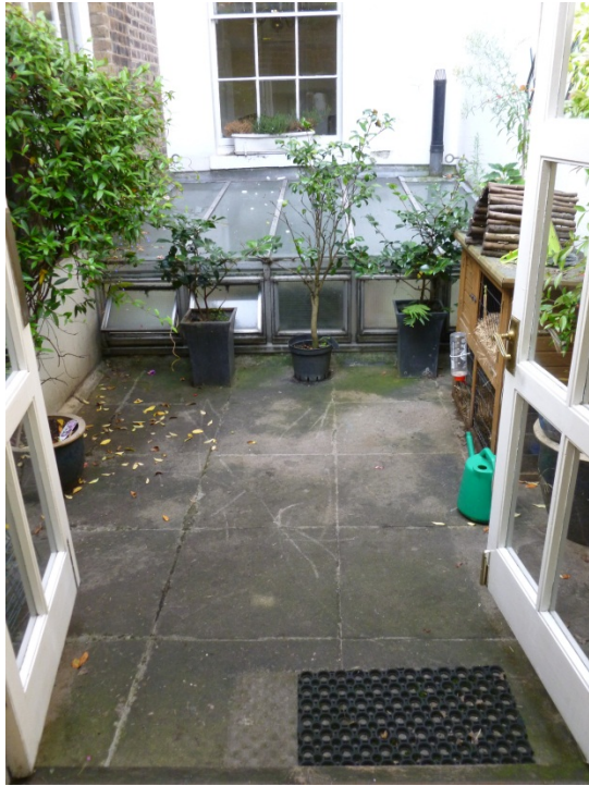
Existing courtyard lantern rooflight to be removed to allow for an open courtyard to the basement and the terrace replaced with new including an obscure glazed floor as indicated on the drawings.
