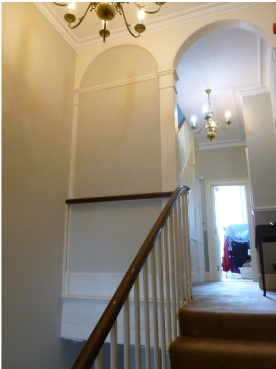
Existing second floor infill panel to be removed and replaced with a clear glazed window.
