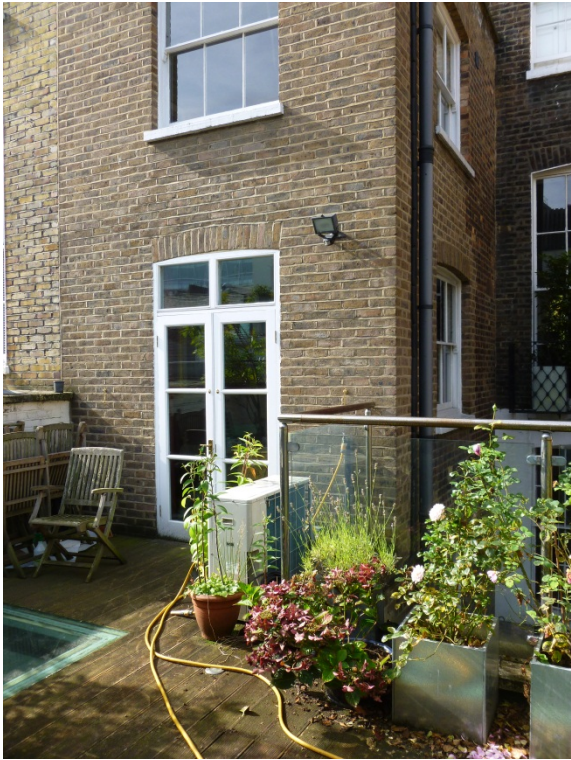
Existing first floor external door to be replaced with a new painted timber door to accommodate new terrace level.
