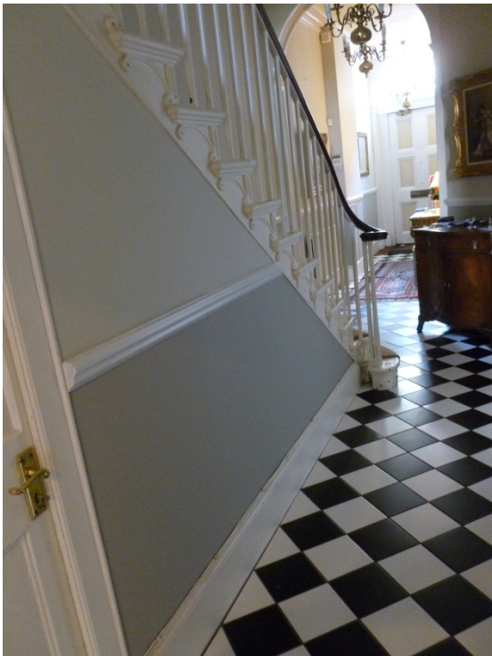
Existing ground floor staircase, original balusters and handrail behind the panel below the stair to be exposed.
