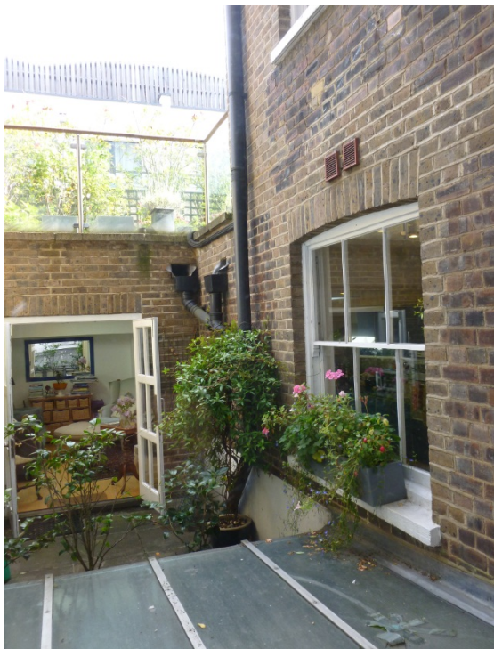
Existing courtyard timber doors and windows to be removed for new openings as indicated on the drawings.
