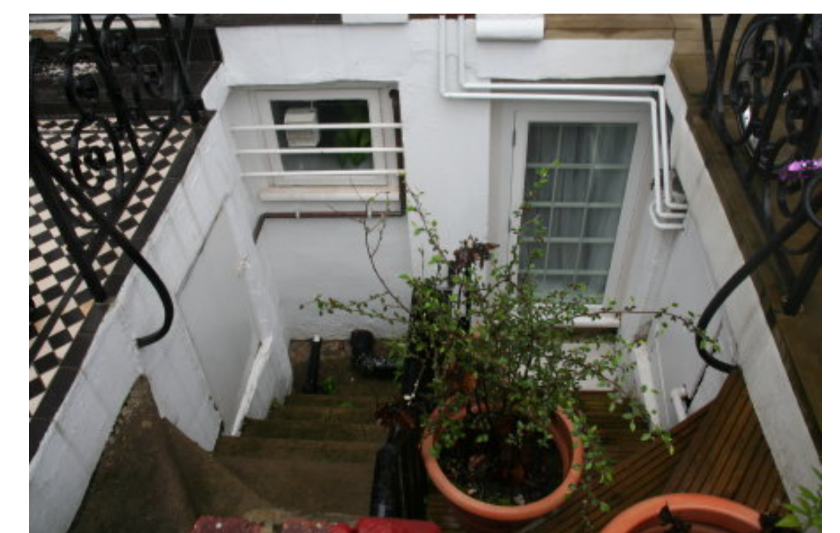
Photo 3: view of the front area steps and basement windows to nos. 41 (left) and 43 (right) Howitt Road.
