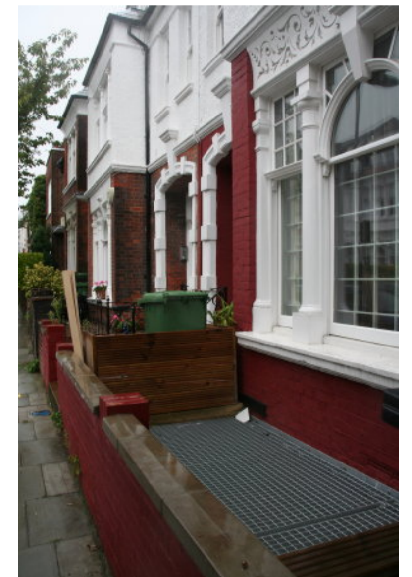
Photo 5: view of the front area of no. 43 Howitt Road, showing the white steel grille above an existing lightwell serving basement windows. no. 41 is to the left.
