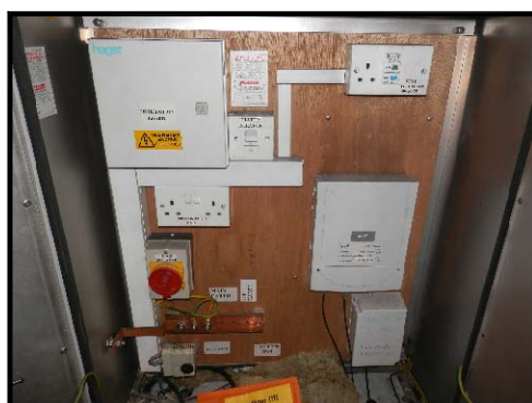
VIEW D – EXISTING DISTRIBUTION BOARD LOCATION
