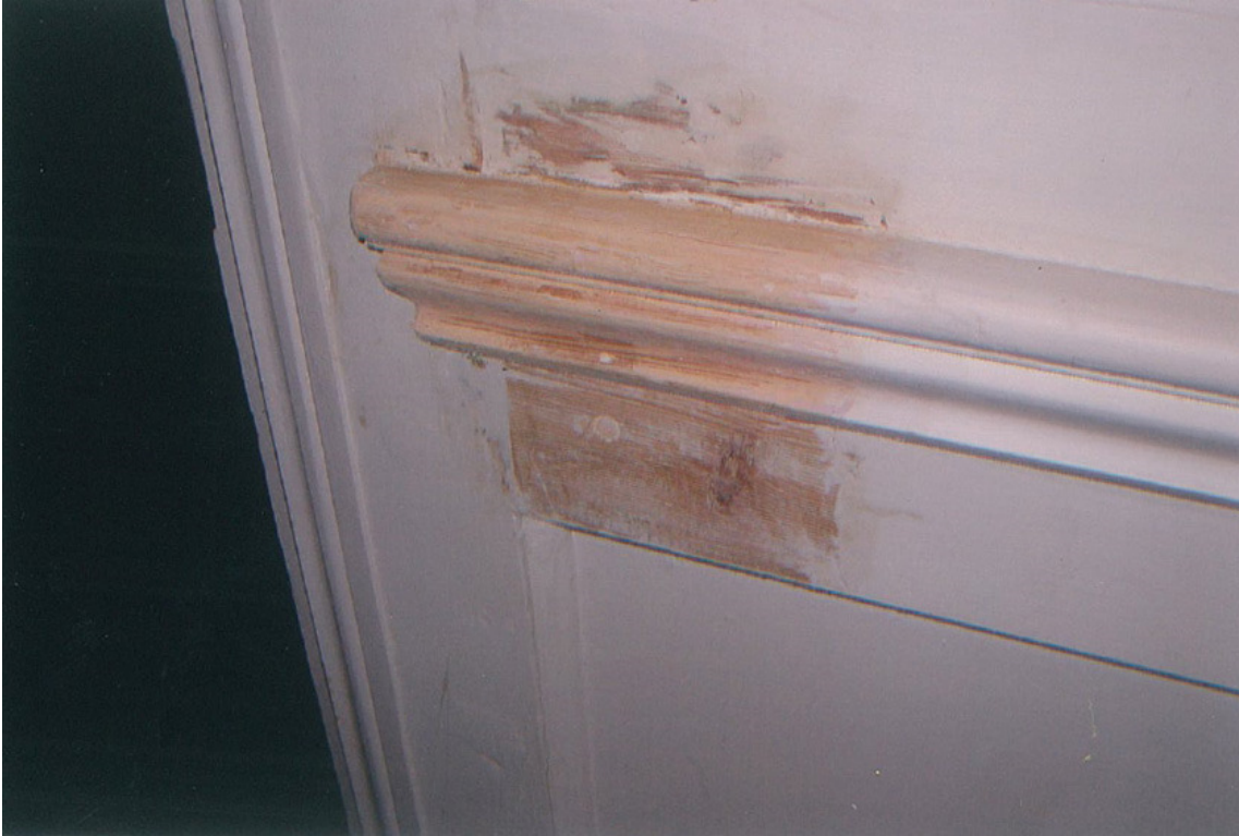
Dado rail to north wall of ground floor rear room: Revealed modern joinery
