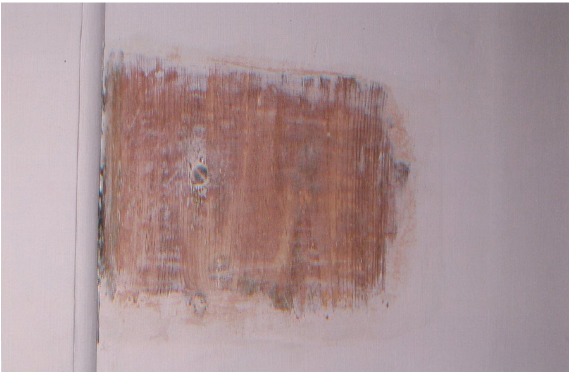
Paint investigation on panel field of north wall of ground floor rear room: Revealed modern joinery
