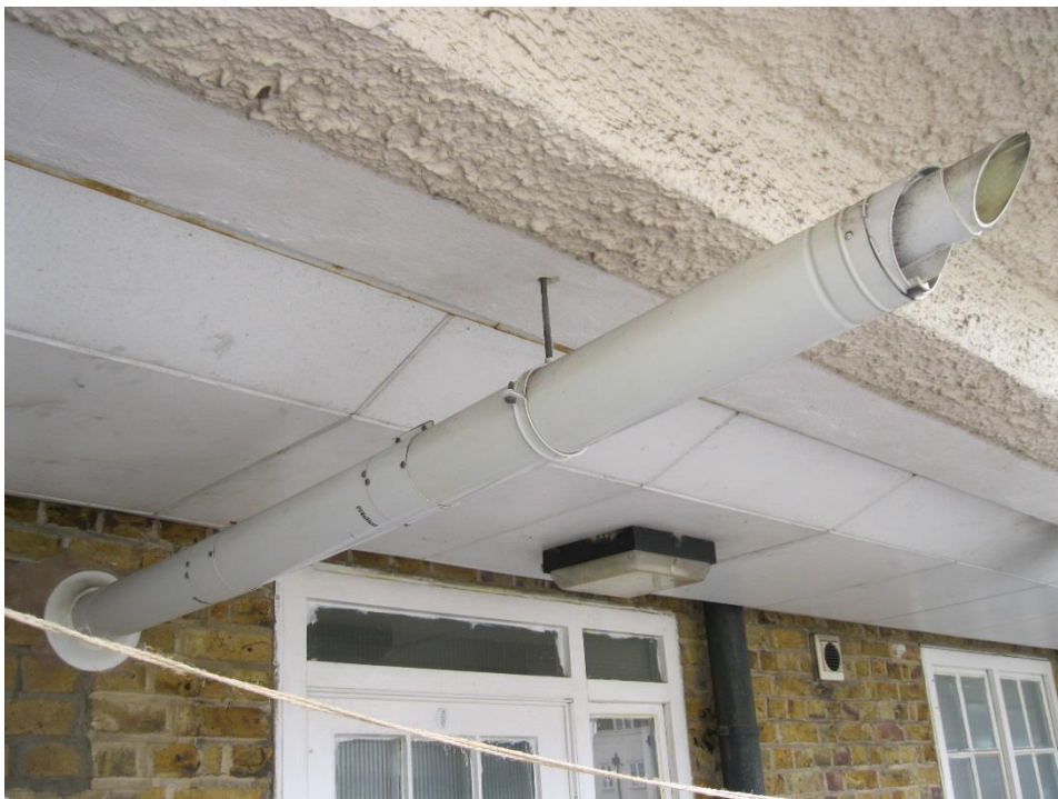
Photograph 6 Typical boiler flue on access balcony
