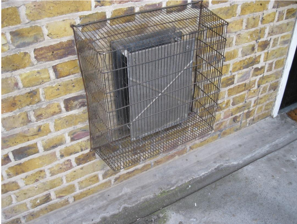
Photograph 5 Typical balanced flue terminal on access balcony
