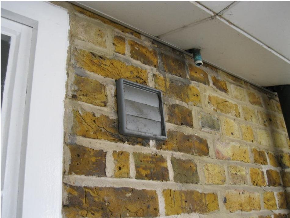
Photograph 2 Alternative but typical fan terminal
