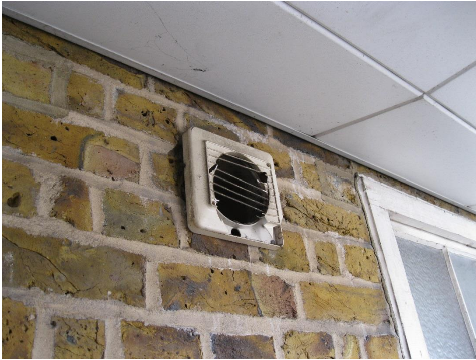
Photograph 1 Typical WC/Bathroom fan terminal on access balcony
