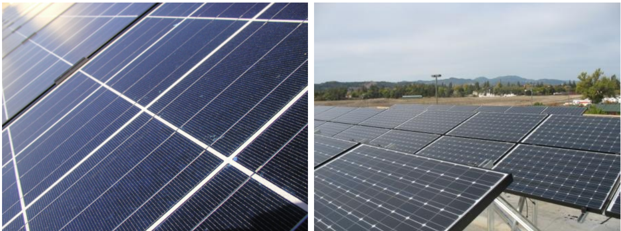
Figure 3 - Typical photovoltaic panel installations
