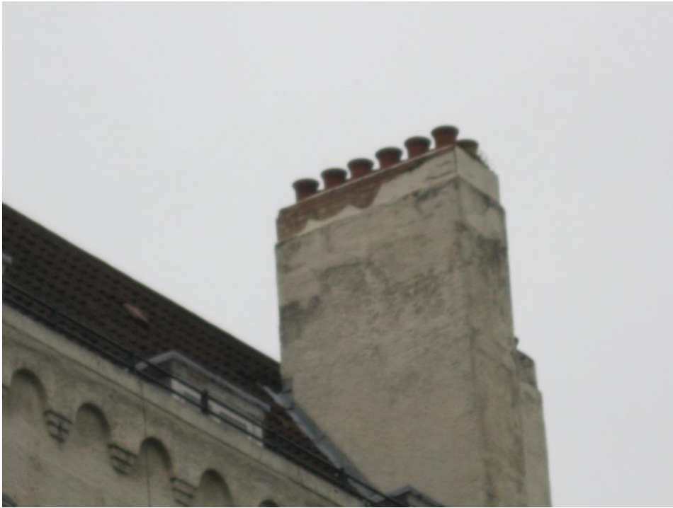
Photograph 5 Chimney defective render - rear
