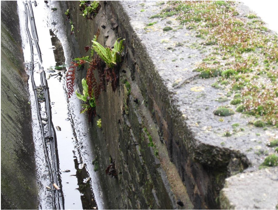
Photograph 9 Parapet wall and gutter vegetation growth
