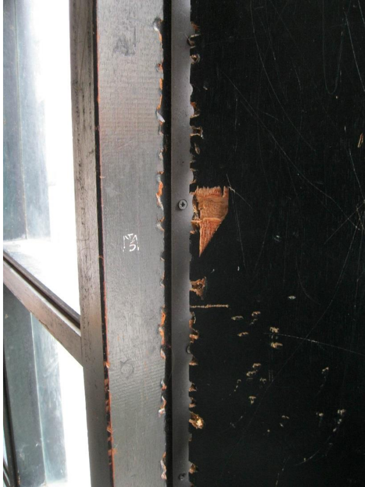
Photograph 18 Damage to communal door leaf
