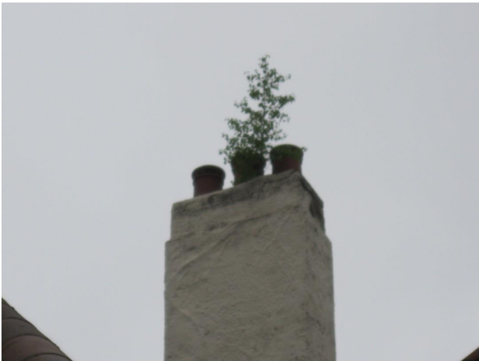
Photograph 6 Chimney – vegetation growth
