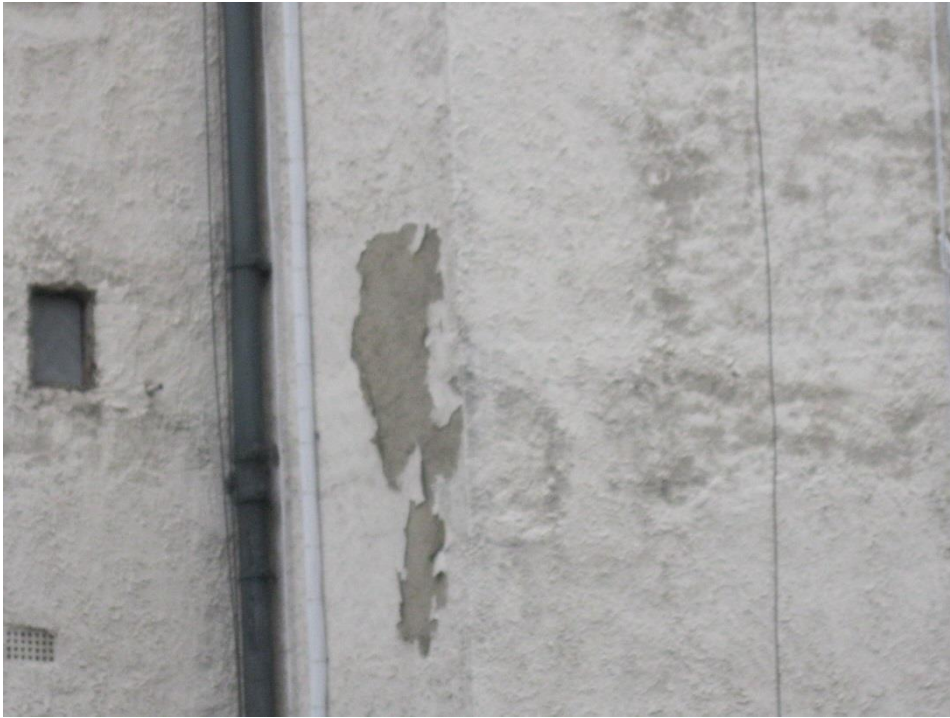
Photograph 7 Render – defective coatings
