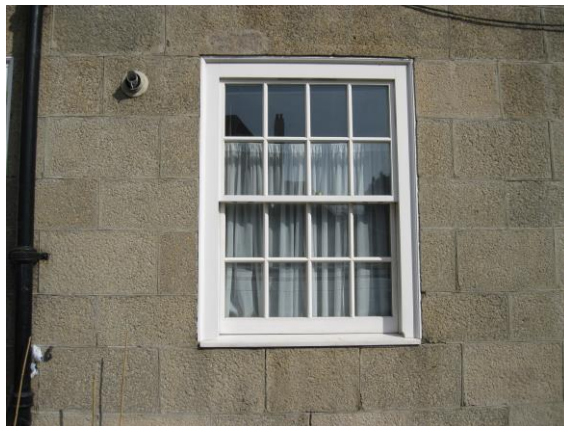
Proposed replacement timber window type as fitted in adjacent part of Levita House
