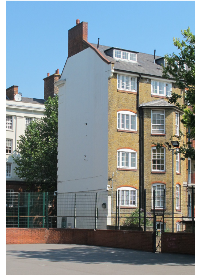
Gable end wall of Nigel building showing gable wall and chimney to be built up.
