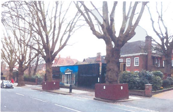
Photographs 2 & 3: Box hoarding around plane trees T1, T2 and beech tree T7
