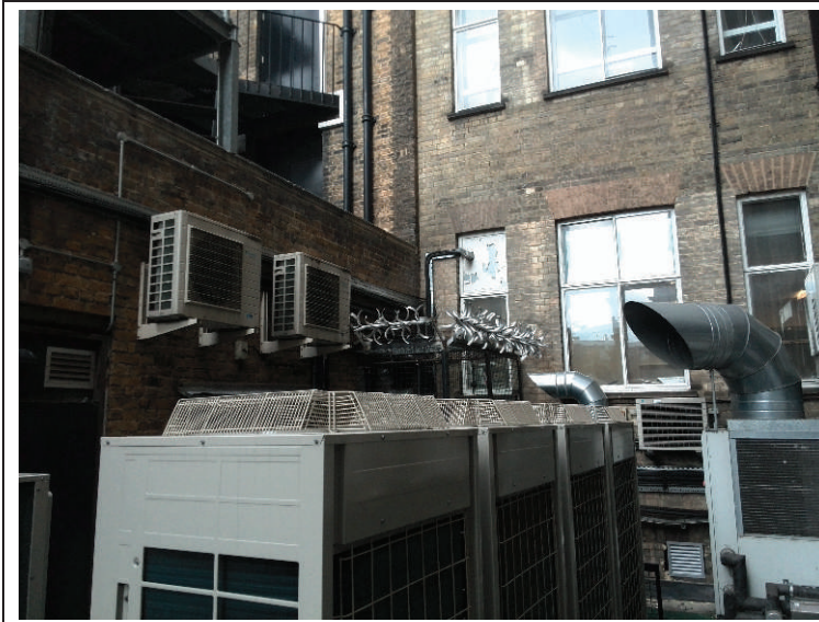
View facing north east towards the existing plant on the roof above the Physics building entrance. Photograph taken on the 26.09.2014.
