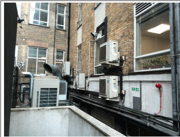
View facing east towards the wall where the new condenser unit is positioned. Photograph taken on the 26.09.2014.
