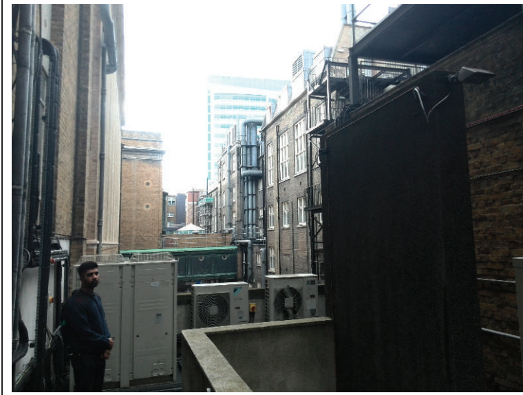
View facing west out over the roof plant into the courtyard adjacent to the Physics Building rear entrances. Photograph taken on the 26.09.2014.
