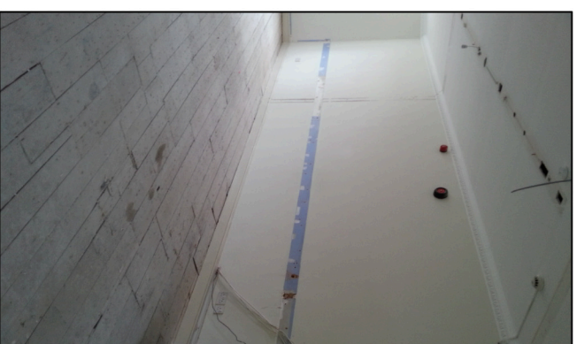
F Third floor photographs displaying hallway floor. - (existing carpet tiles removed) Boards retained - to be re-carpeted
