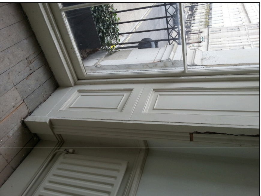
A First floor photographs displaying existing floor. Boards retained - (existing carpet tiles removed) To be re-carpeted
