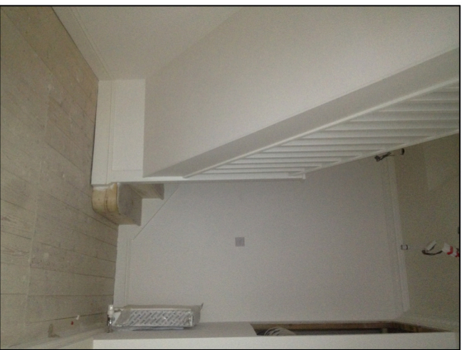
D Second floor photographs displaying hallway floor. - (existing carpet tiles removed) Boards retained - to be re-carpeted
