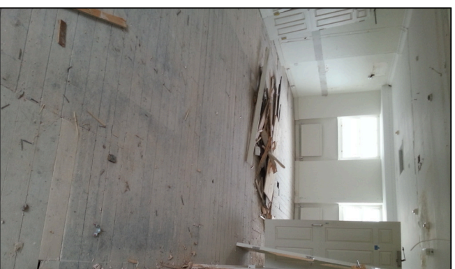
G Third floor photographs displaying hallway floor. - (existing carpet tiles removed) Boards retained - to be re-carpeted
