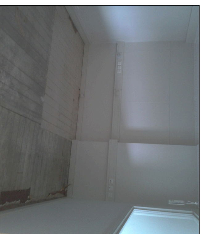
H Third floor photographs displaying hallway floor. - (existing carpet tiles removed) Boards retained - to be re-carpeted
