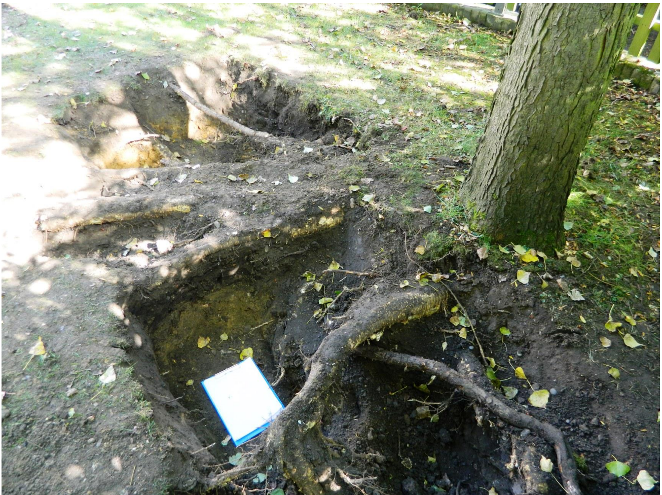
Figure 1. Exposed structural roots of T5. The edge of the roof slab of the existing underground garage is level with the right hand edge of the clipboard, i.e. 600 mm away from the trunk.
