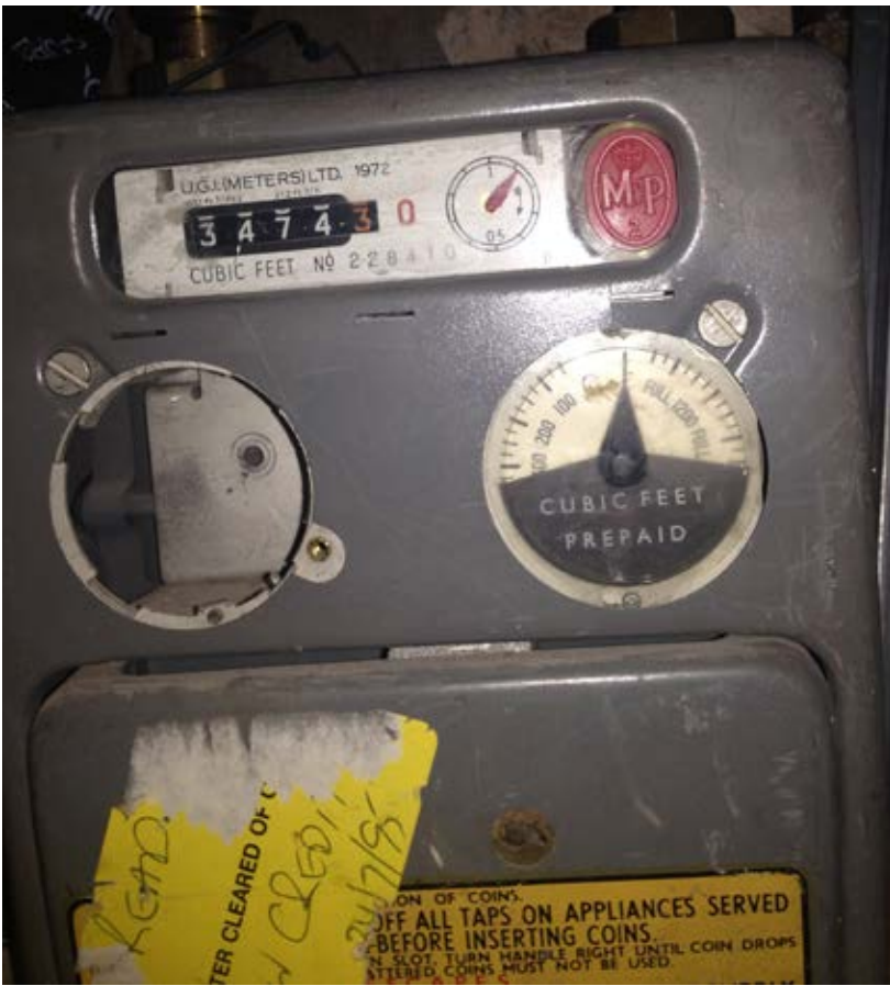
Photograph of existing gas meters to second floor flats
