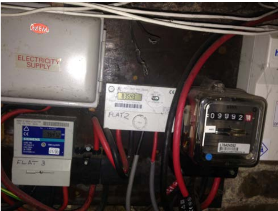
Photograph of existing electricity meters to ground, first and second floor flats
