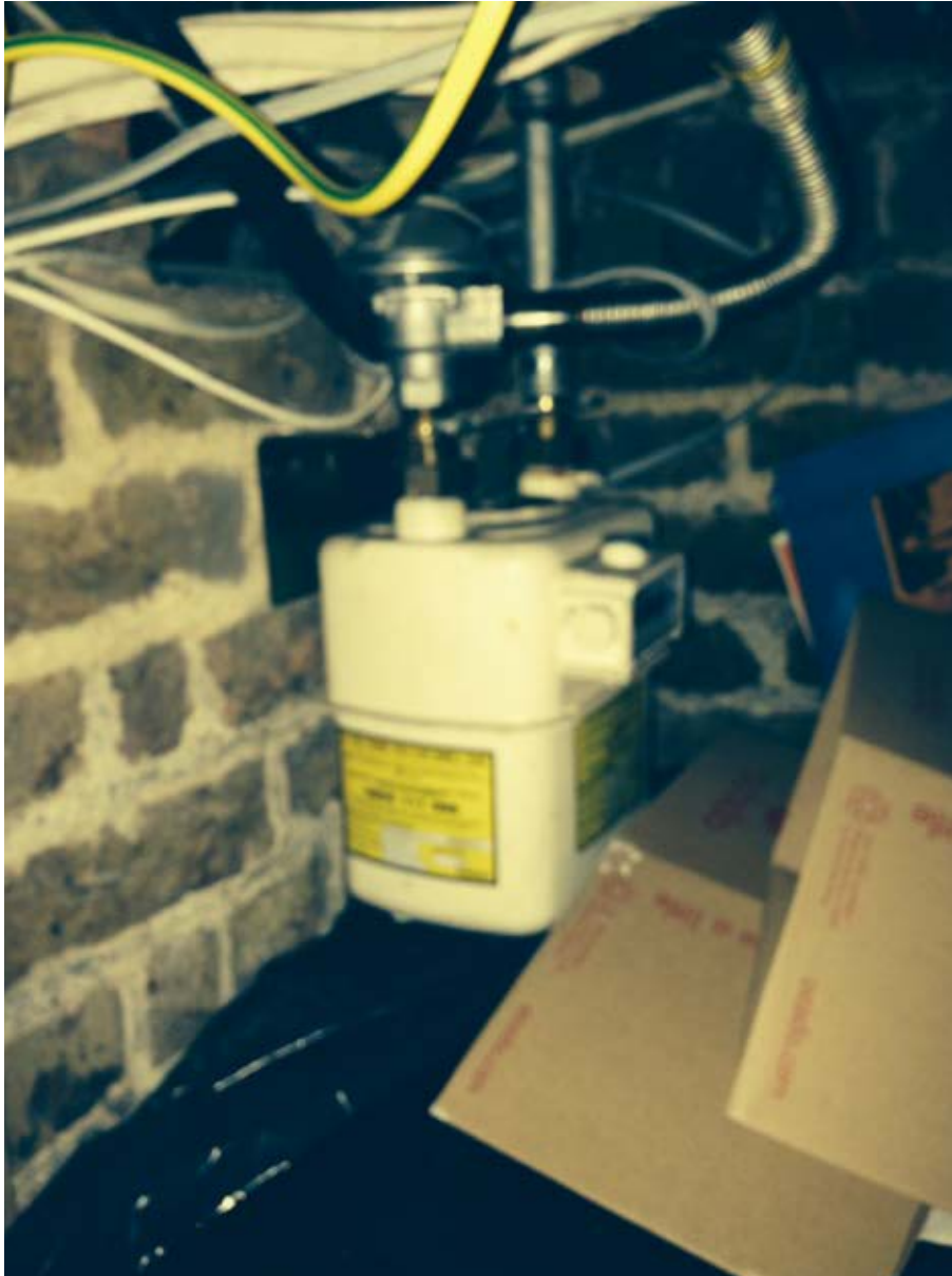
Photograph of existing gas meter to ground floor flat
