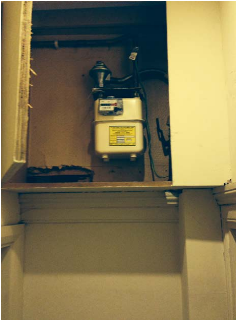
Photograph of existing gas meter to first floor flat
