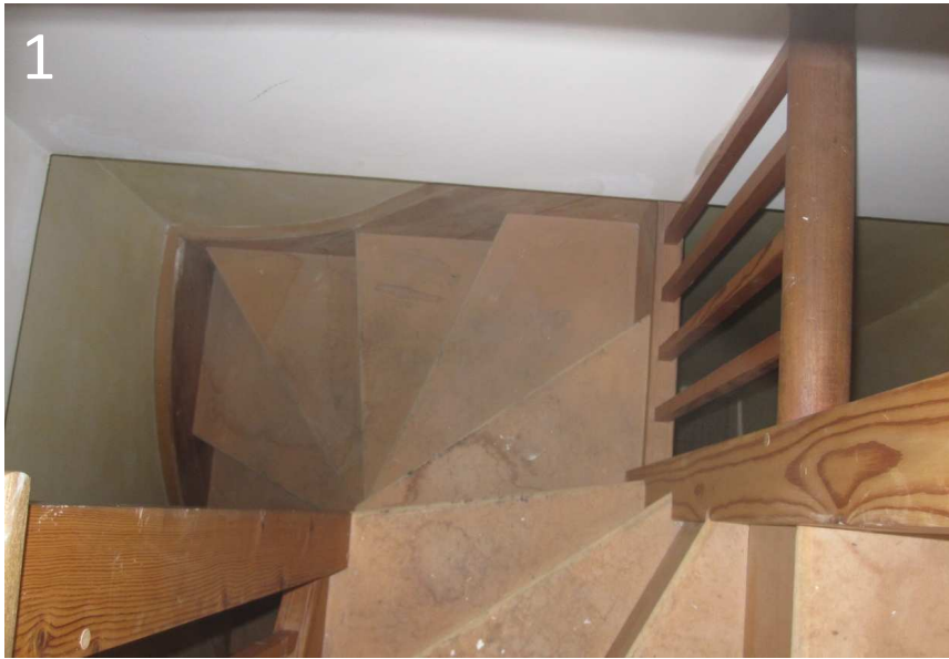
1 View from the top of the wooden roof access stair, showing treads
