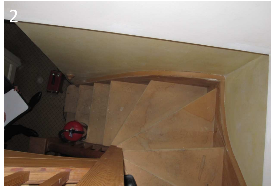
2 View from the top of the wooden roof access stair, showing treads
