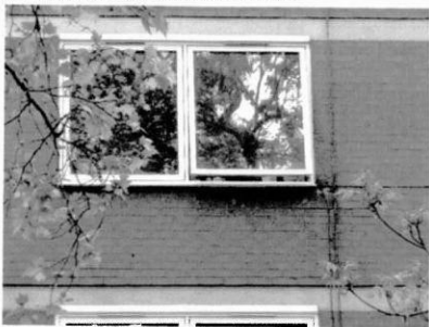
Photograph 3 – Close view of Flat 18 – No weeps holes visible.
