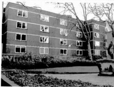
Photograph 2 – West Elevation, arrows point to locations where bricks were removed.
