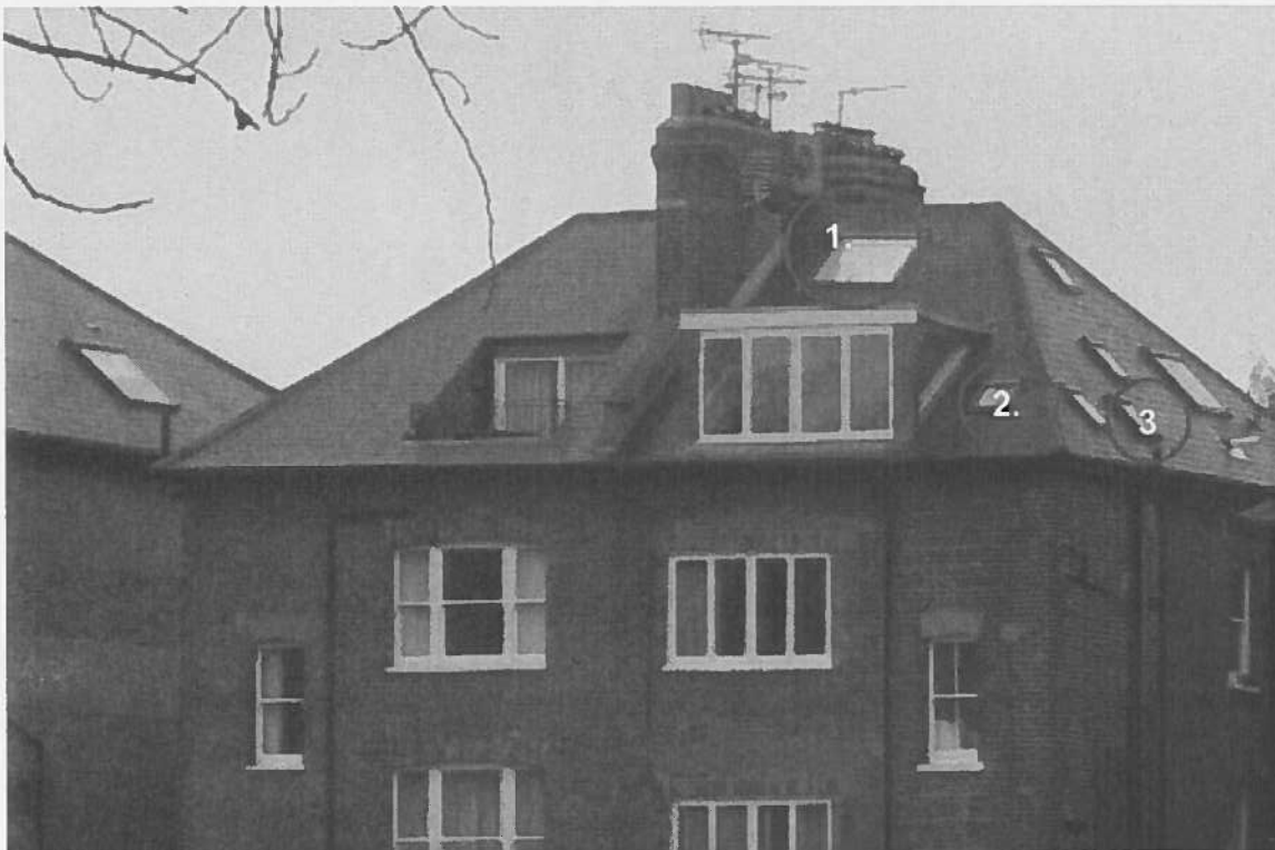
Rooflights subject to the enforcement notice.
