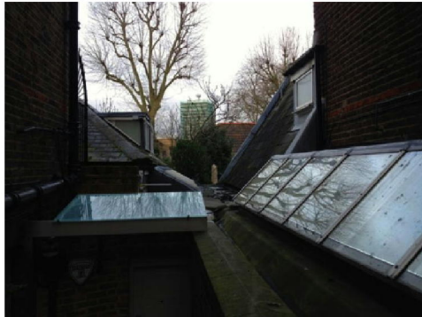
CLOSE UP VIEW OF GAP BETWEEN NOS. 76 & 74
