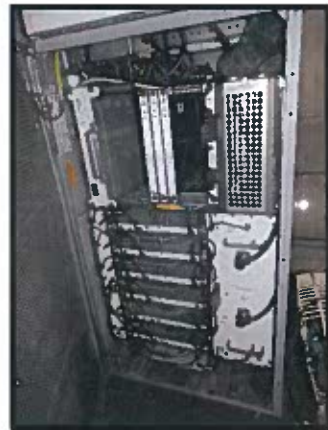
VIEW B – EXISTING 2G EQUIPMENT LOCATION
