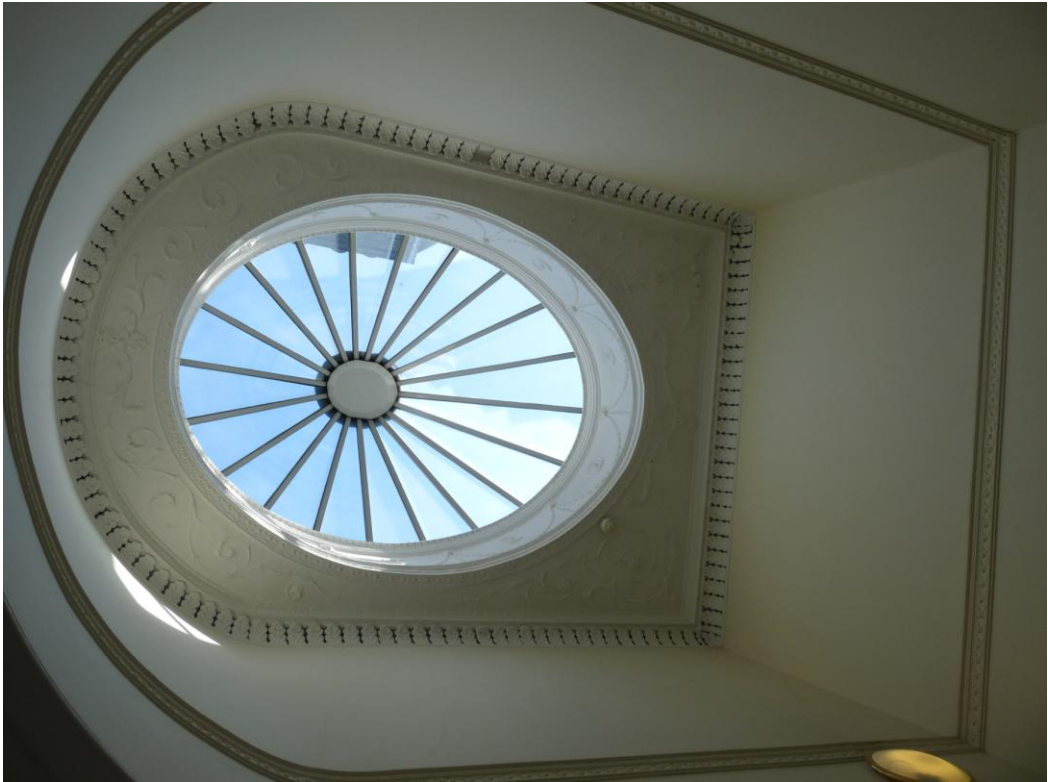
Rooflight to main staircase
