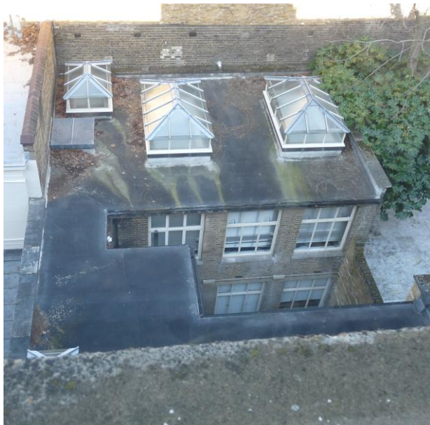
Roof top view of existing back wing. Note concrete cill to back closet wing in foreground
