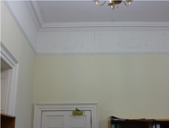
9. Differential movement and cracking between stair and timber stud wall.
