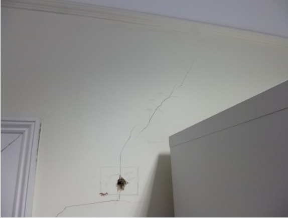
1. Movement and cracking of timber stud wall at 2 nd floor level.
