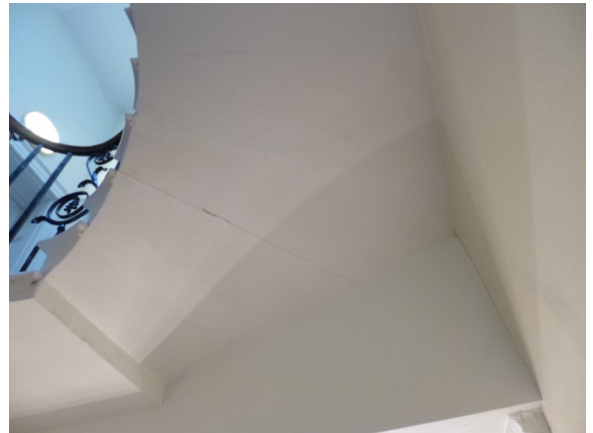
10. Hairline cracking to underside of stair.
