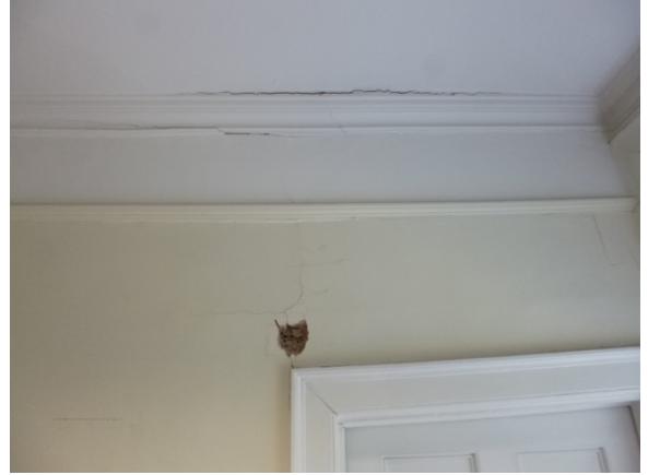
2. Movement and cracking of timber stud walls at 2 nd floor level.
