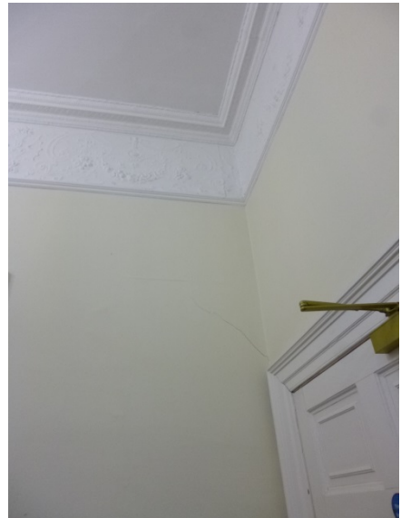
8. Movement of timber stud walls/floor.
