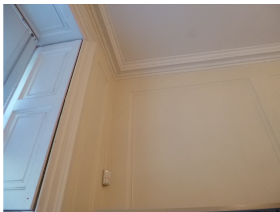
11. Differential movement between hall wall and front wall at ground floor level.
