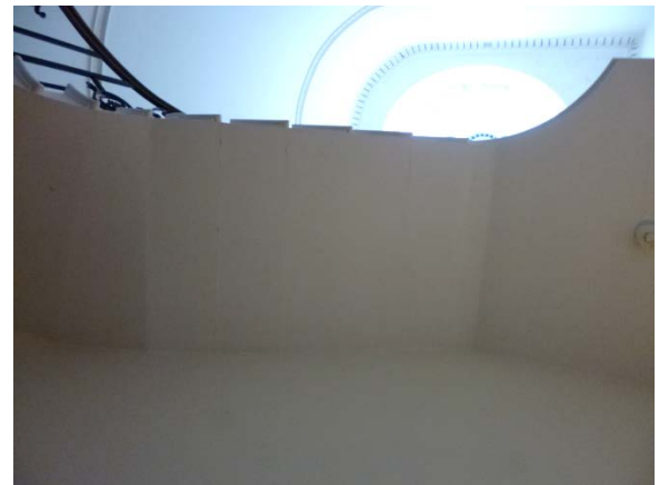
4. Hairline cracking of stone stair treads.
