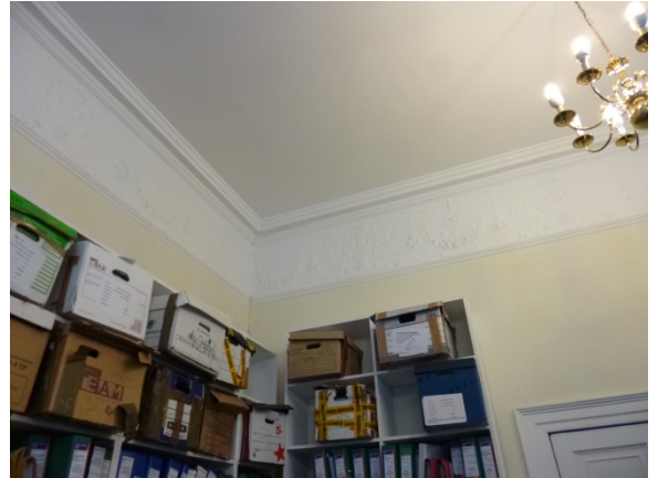
6. Differential movement between spine wall and party wall at first floor level.
