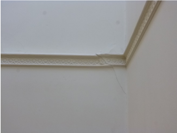
5. Cracking and differential movement between internal spine wall and party wall.
