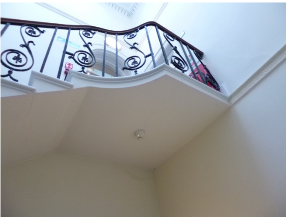
3. Hairline cracking of stone stair.
