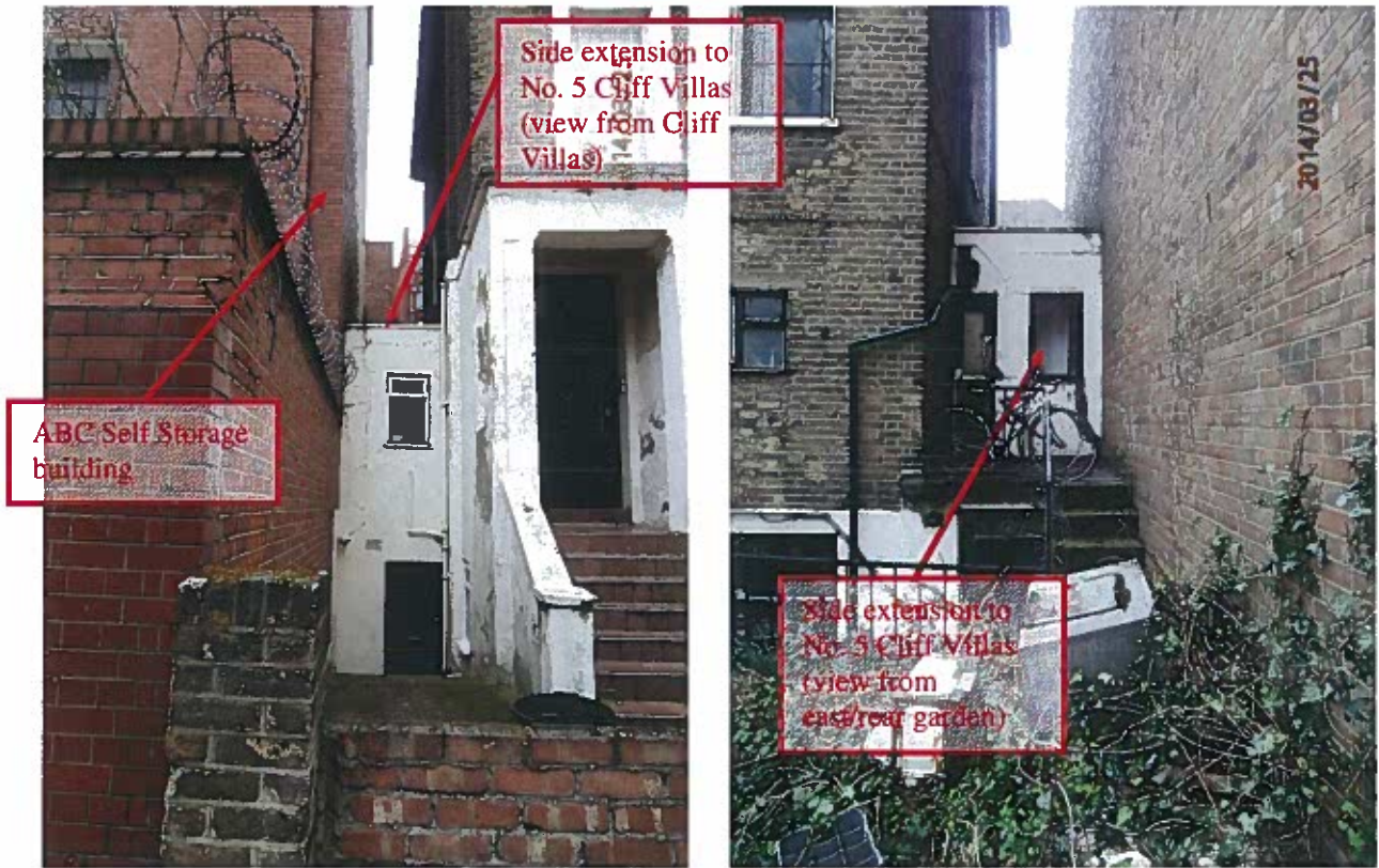
Figure 2 - North boundary of property where side extension of No. 5 Cliff Villas adjoins storage building
