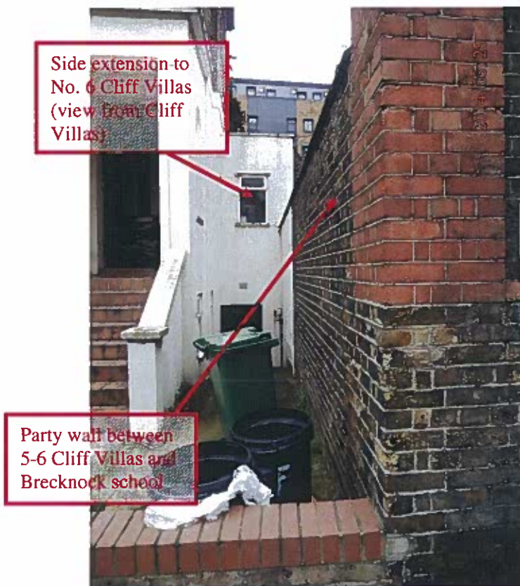
Figure 4 - South boundary of property where flank wall of No. 6 side extension appears to be on school land
