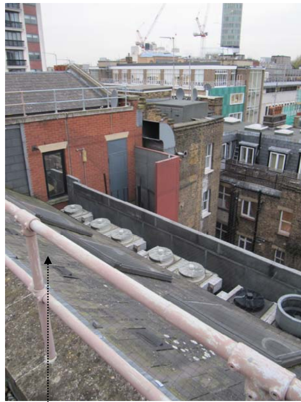
Roof to be lifted to create access to proposed Fourth Floor terrace
