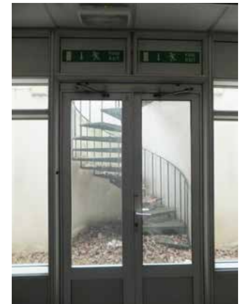
Exit to the existing light well_ Stair connecting basement and ground floor
