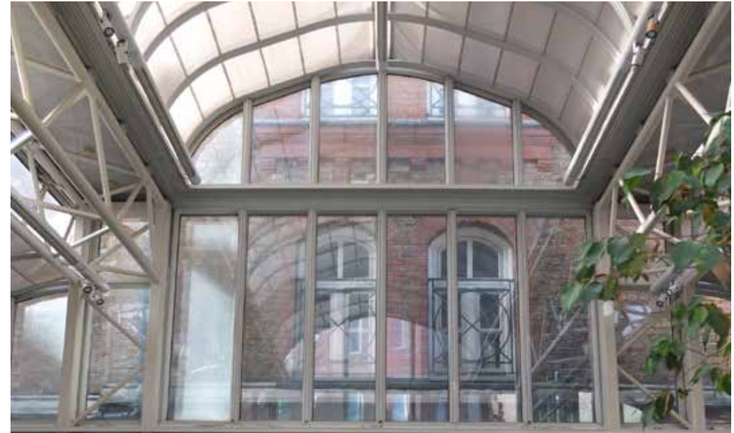
Conservatory and its connection with the existing building. Apart from at the ground floor level it is not attached to the building_Ground Floor.
