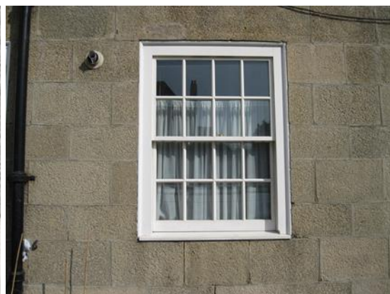
Proposed replacement sash window type as fitted in adjacent Levita House block
