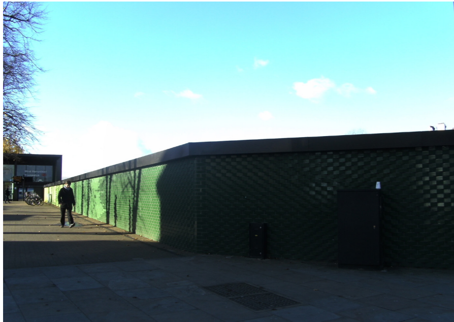
LOCATION WITH POLE Wall to railway cutting at corner of Iverson Road and West End Lane.
