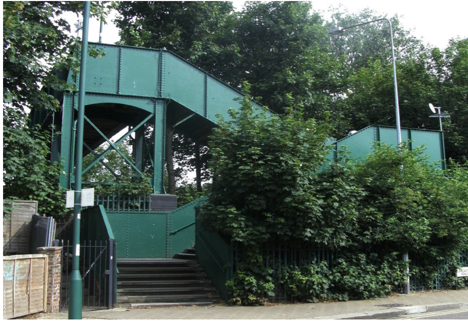
LOCATION WITH POLES Pedestrian bridge on corner of Kendall Road as existing.
