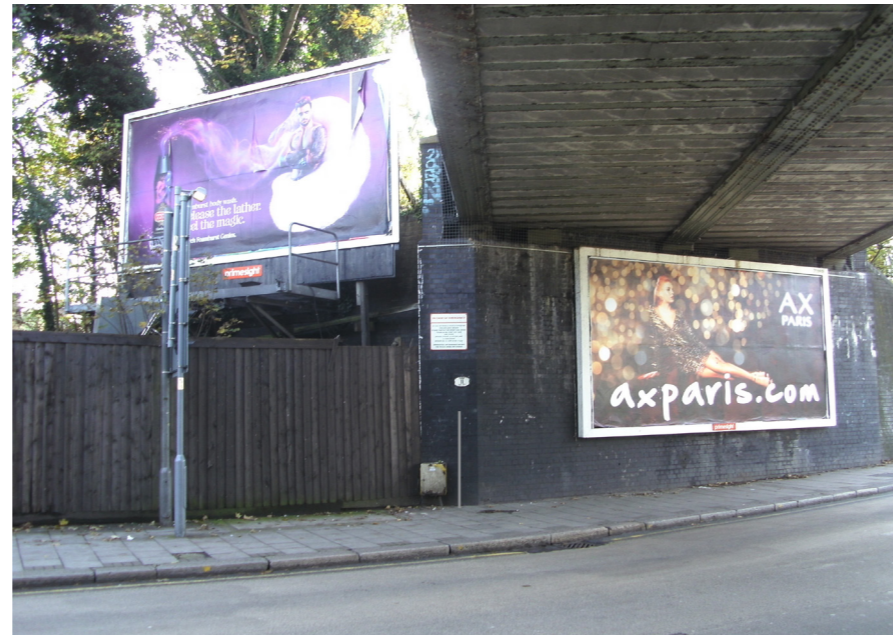
LOCATION WITH POLE East side of south abutment wall of railway bridge over Acton Lane with proposed 1 - metre high black pole 50mm from face of wall, centered under east edge beam of bridge over.
