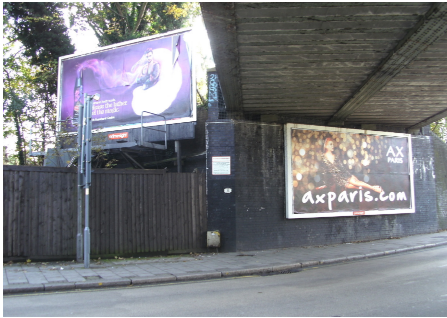
LOCATION WITHOUT POLE East side of south abutment wall of railway bridge over Acton Lane.
