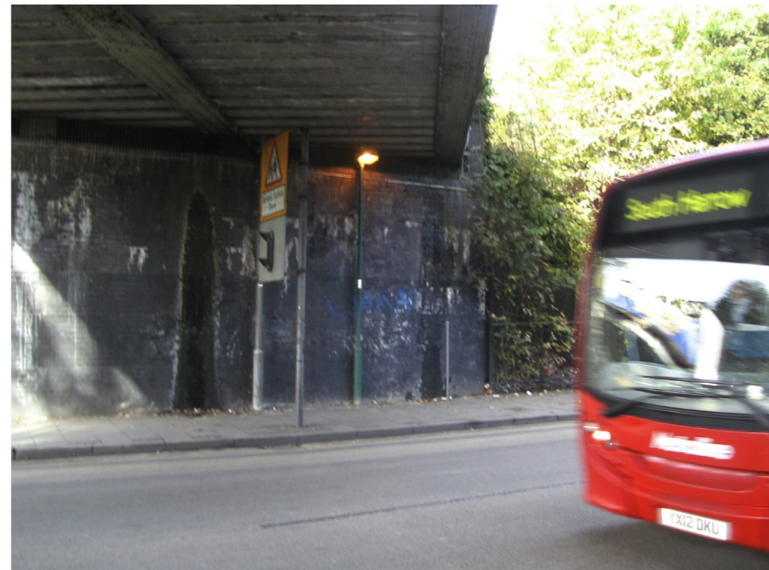
LOCATION WITH POLE East side of north abutment wall of railway bridge over Acton Lane with proposed 1 - metre high black pole 50mm from face of wall, centered under east edge beam of bridge over.
