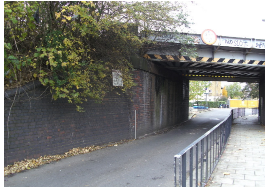
LOCATION WITH POLE South abutment of railway bridge with proposed pole under east girder of bridge over.
