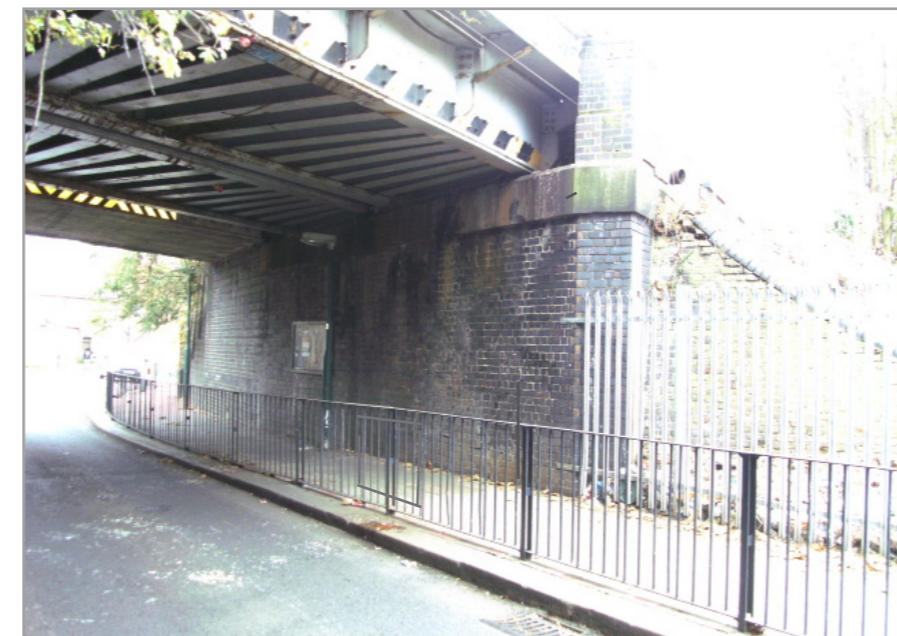
LOCATION WITH POLE North abutment of railway bridge with proposed pole under east edge girder of bridge over.
