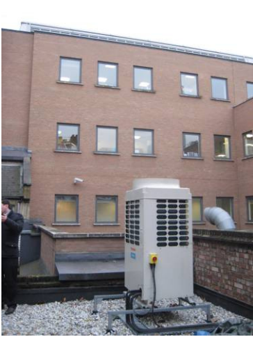
Existing condenser unit
