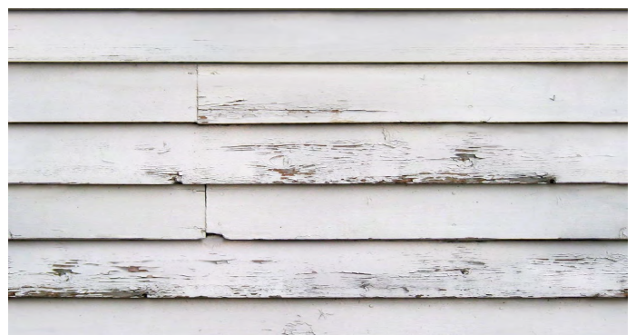
Example of painted horizontal timber boarding for the new bin & bike store.
