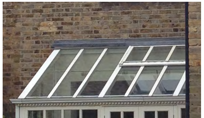
Example of a glazed roof proposed for the new bin & bike store.
