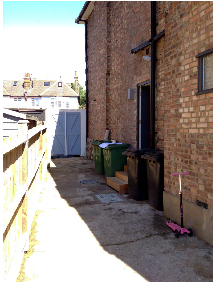
The existing side elevation showing the space to accommodate the proposed new store.
