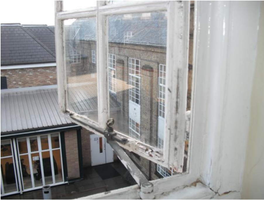
PHOTO 2 CONDITION OF EXISTING SINGLE GLAZED STEEL WINDOW.
