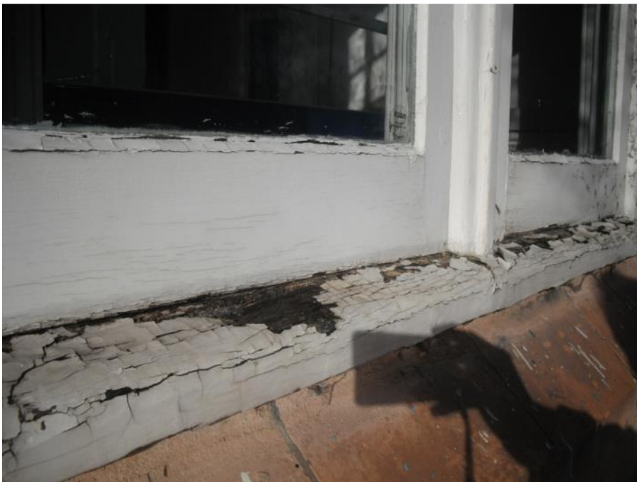
PHOTO 1 CONDITION OF EXISTING SINGLE GLAZED TIMBER WINDOW
