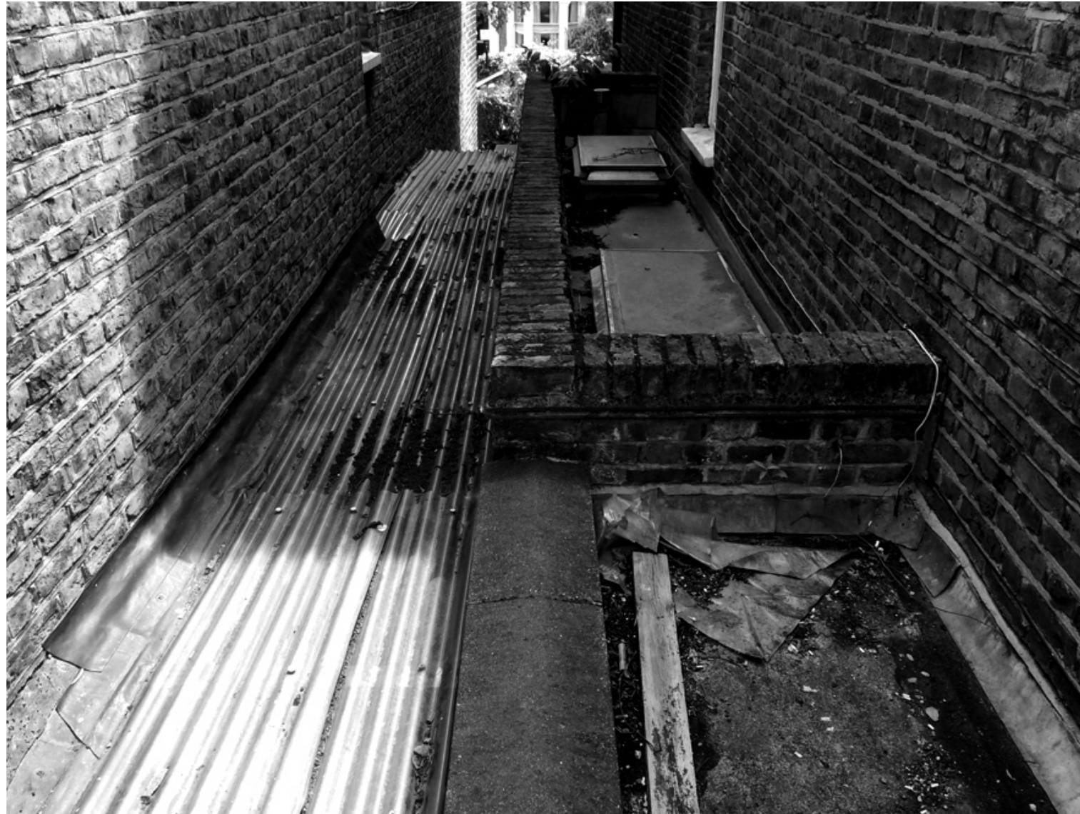
View of alley way between No52 (on the left) and No54 looking towards the street
