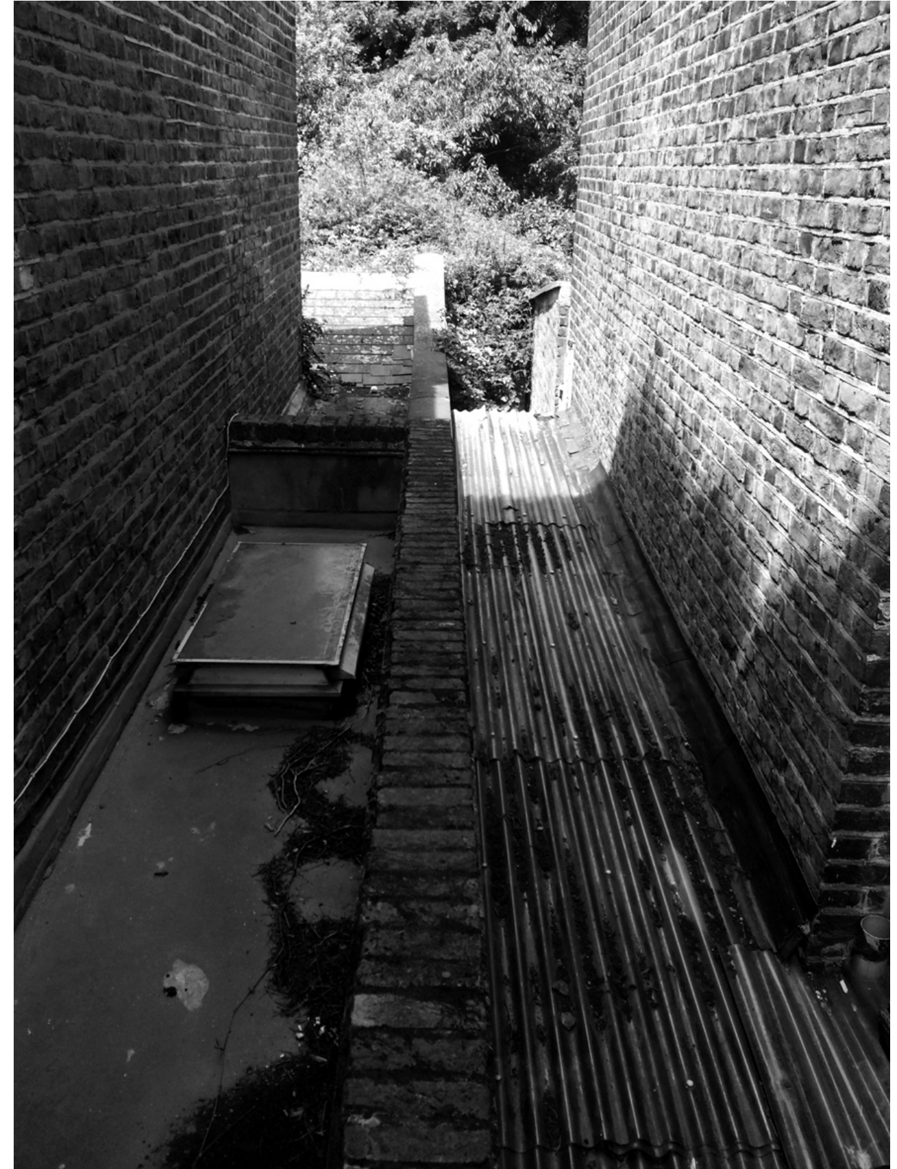
View of alley way between No52 (on the right) and No54 looking towards the garden
