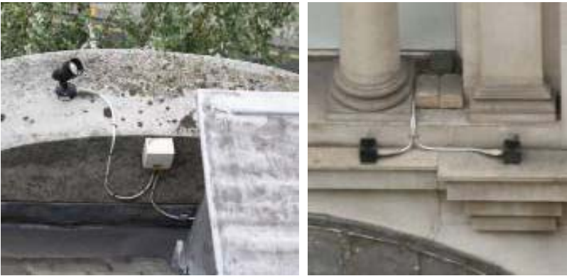
Spotlights anchor-bolt mounted onto stonework with gear boxes tucked out of view
