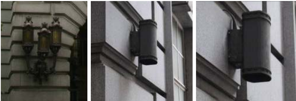
Decorative lanterns and sconces either have rear-entry power feed or top entry with cabling tucked in the grooves of the stonework
