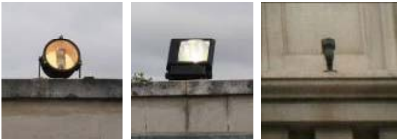
Left to right: Spotlights onto tower, floodlights onto tower, tower uplights
