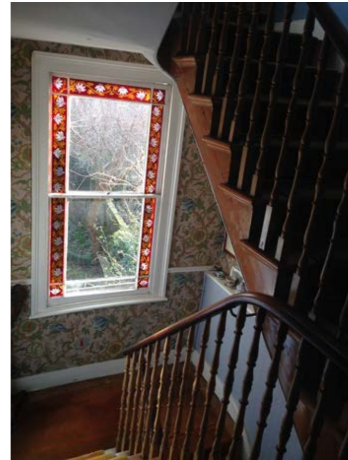
THE ROOF OF THE PROPOSED EXTENSION WILL MEET THE EXISTING PROPERTY LOWER THAN THE WINDOW IN ORDER TO RETAIN THIS ORIGINAL FEATURE.
