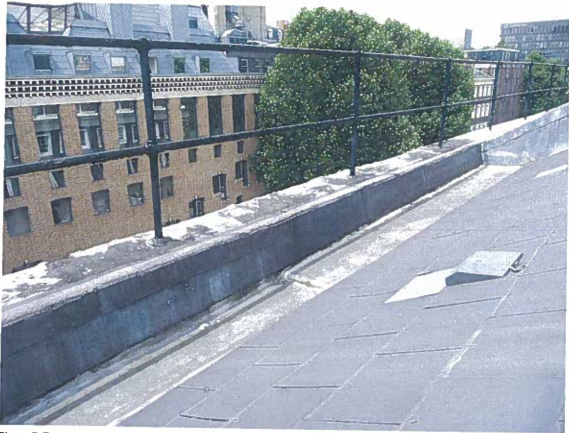
Photo 7: Taviton Annex: Existing guardrails to front elevation.
