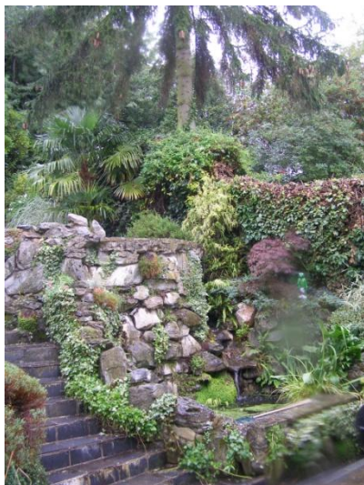
Far Left- the Norway spruce (11) within the garden of 7 Holly Lodge Gardens with its root protection area extending into this garden. Left- the tree is close to the terrace and the retaining walls-any works within the vicinity of the tree should be carried out by hand.
