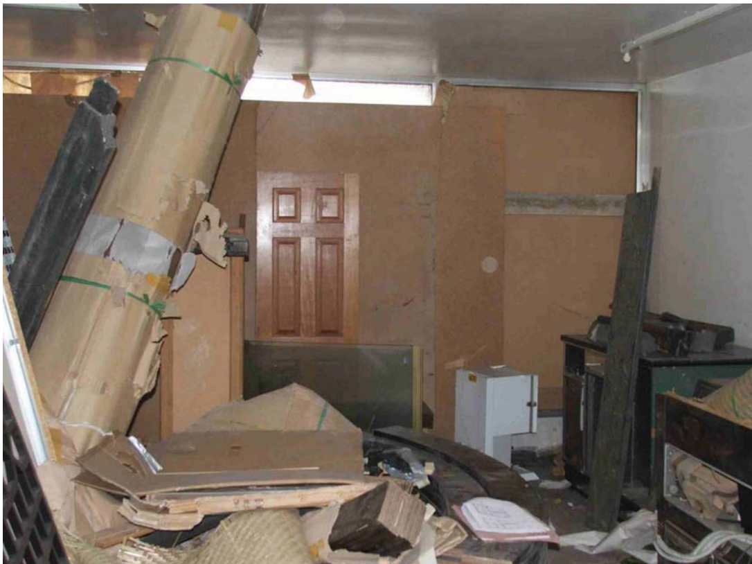
Figure 3.2: View of former shop (boarded shop-front windows)
